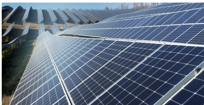
SMART PHOTOVOLTAIC POWER STATIONS – INSTALLATION, MAINTENANCE AND MANAGEMENT
